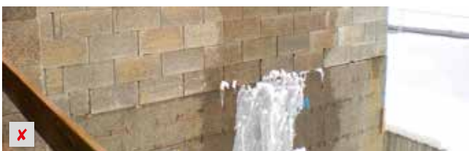
Vlažni tzv. mantelbeton
